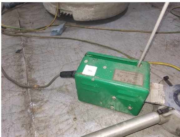
Earthing Switch (ES)
